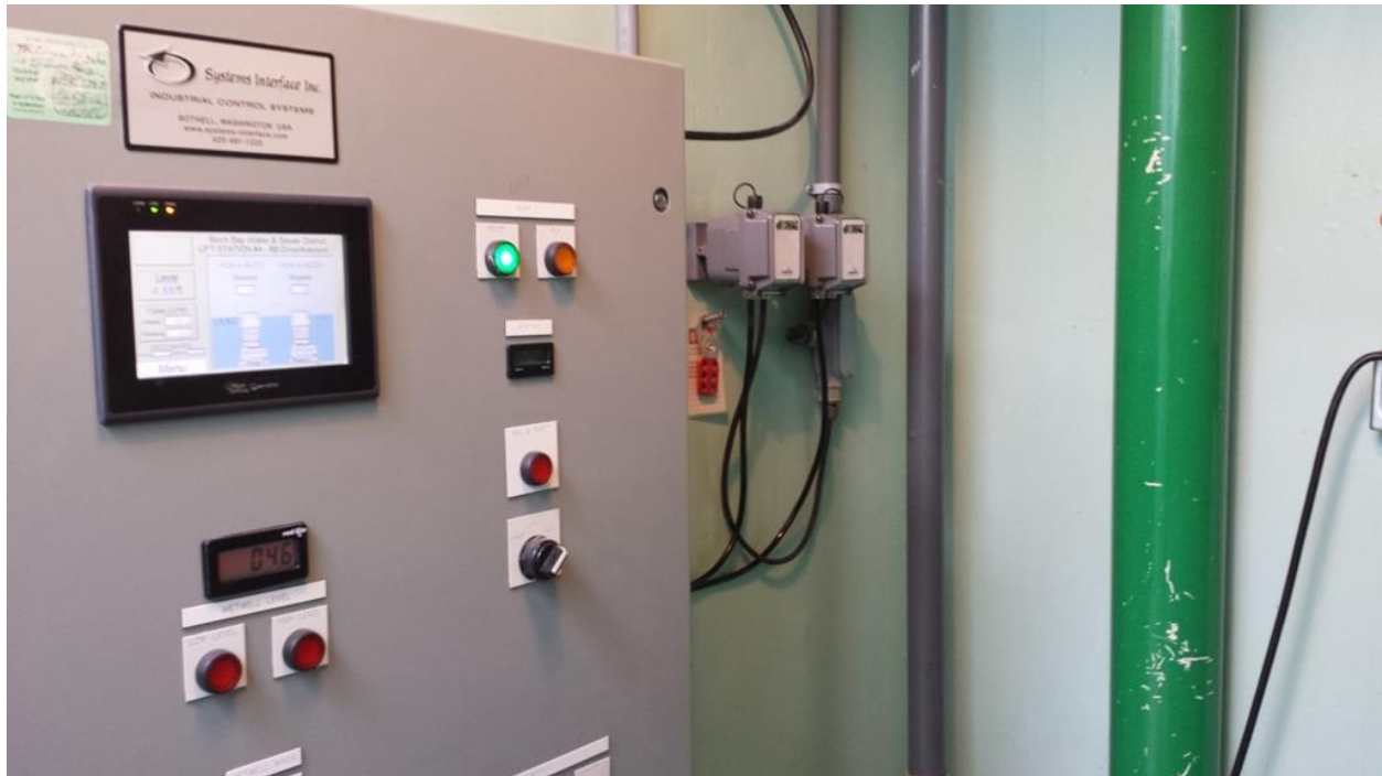
Figure 12 - Control panel and Flow Indicators
