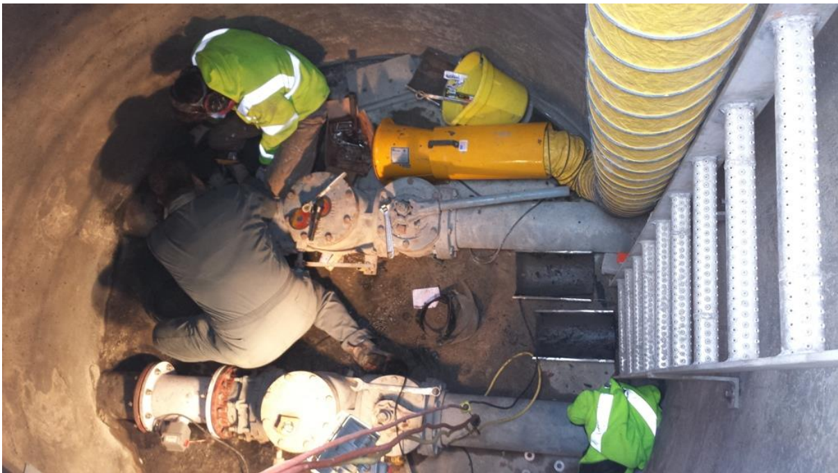
Figure 9 – Crew members installing Seametrics flow meters
