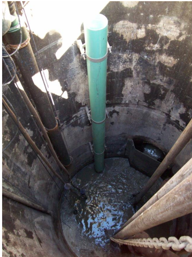
Figure 6 - Lift Station #4 Wetwell
